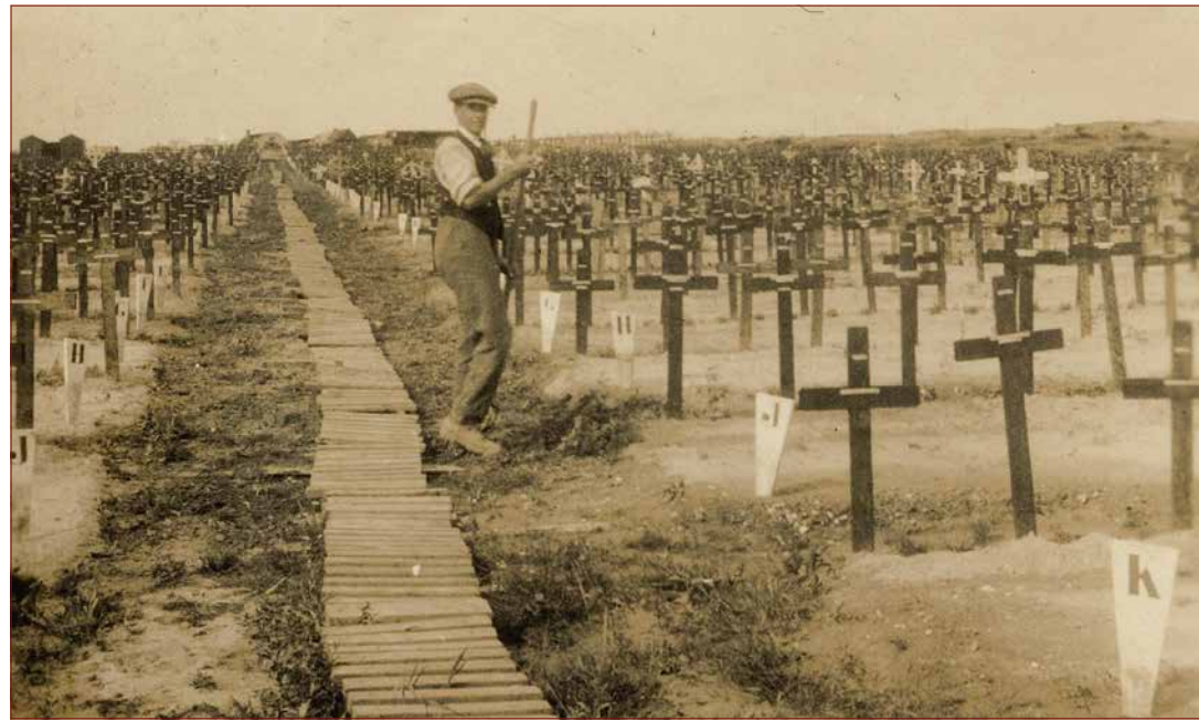
Work on the laying out and construction of Hooze Crater Cemetery, which is just off the Menin Road a couple of miles east of Ypres, is pictured underway at the end of, or just after, the First World War. Note the wooden duck-boards and original IWWG grave markers. Today there are 5,916 Commonwealth servicemen of the First World War buried or commemorated in this cemetery. Of this number 5,730 are unidentified, but special memorials record the names of a number of casualties either known or believed to be buried among them, or whose graves in other cemeteries were destroyed by shell fire. The cemetery was designed by Sir Edwin Lutyens. (Historic Military Press)
