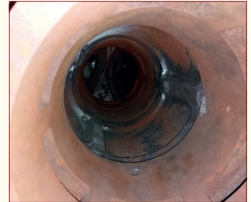
Above: A view into the Valve Chest showing the welded in Port Bars before machining.
