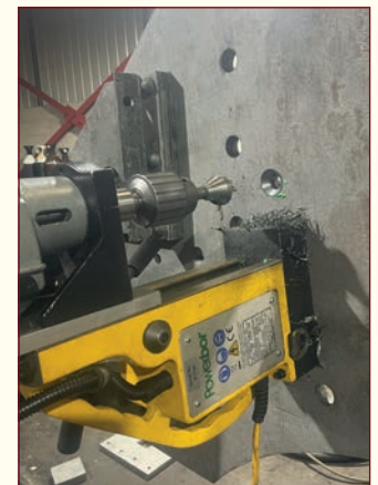
Above: Drilling and countersinking mounting holes for the Front Buffer Beam. PHOTO: PRCLT
