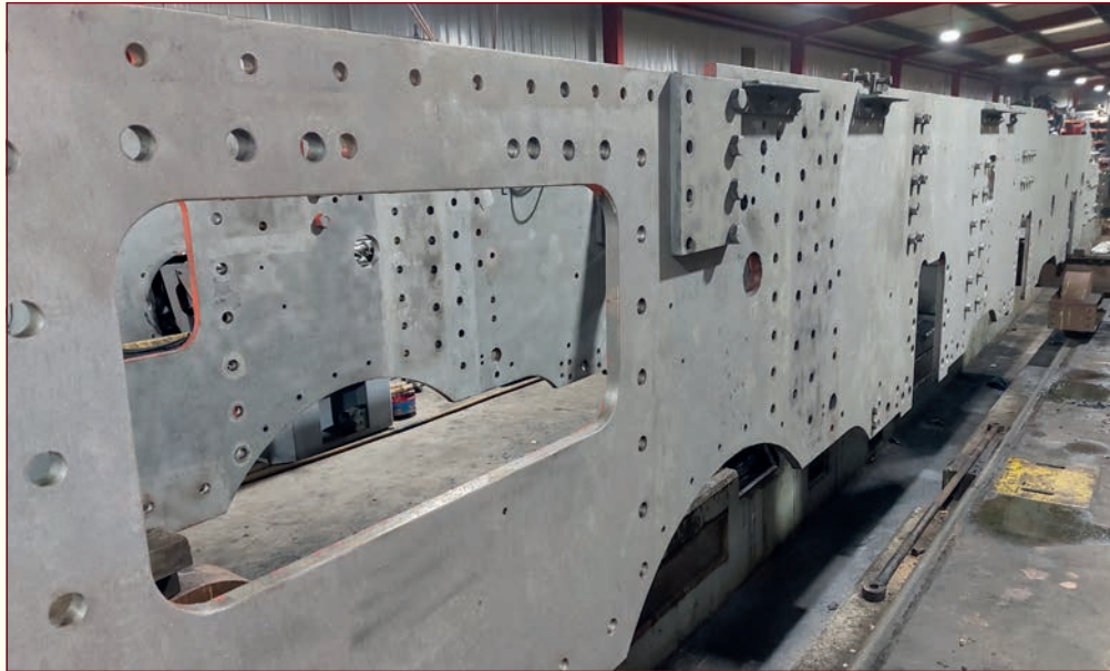
The Chassis of 5551 at West Shed following shot blasting at allow reassembly to restart. PHOTO: KEVIN WEST
